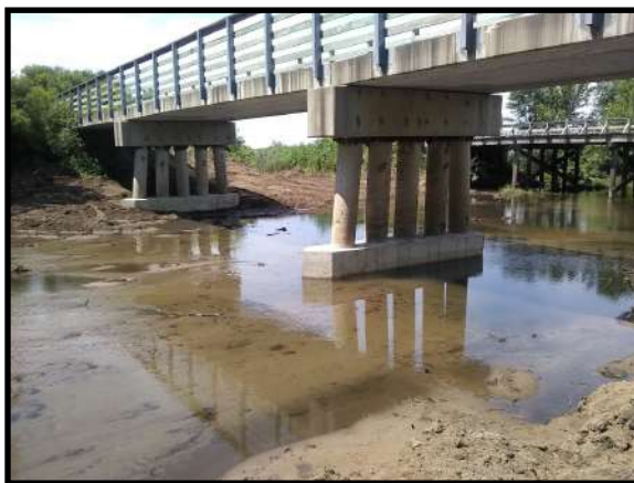
Grump Trail Crane Creek Bridge Pillar Concrete Repair completed by Matt Construction out of Sumner
